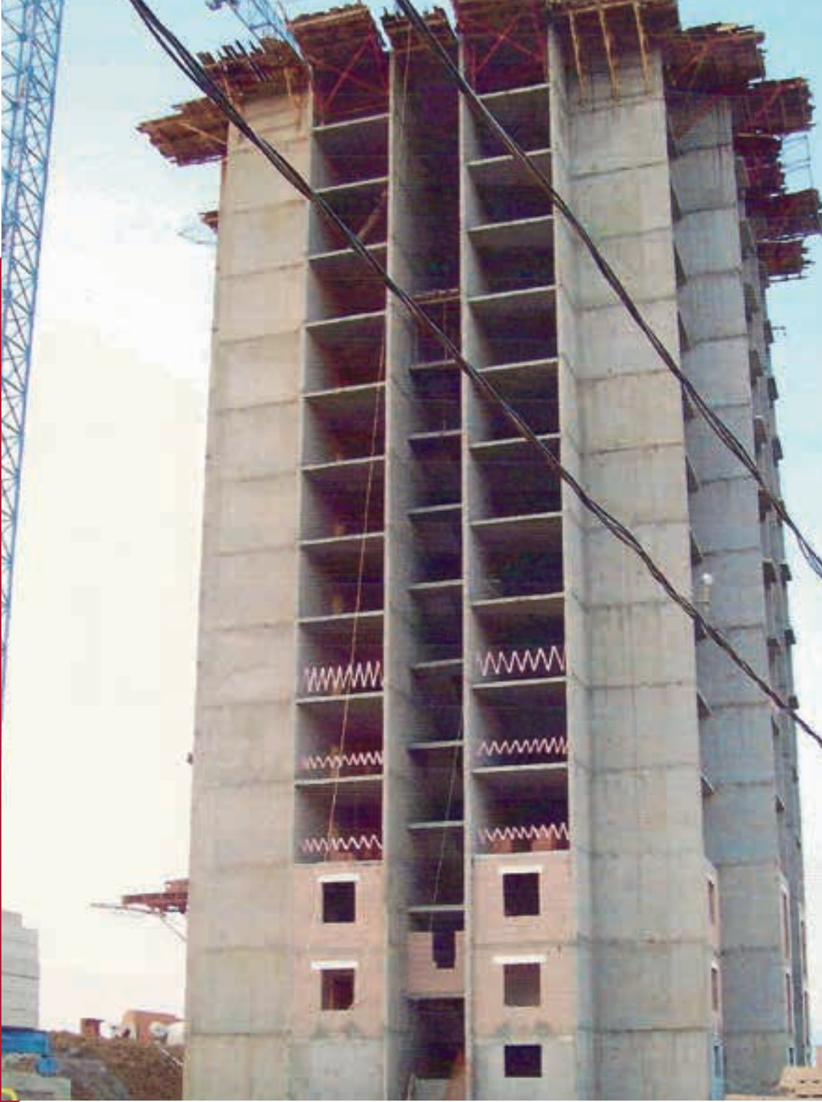
KIPTAŞ BÜYÜKÇEKMECE-TEPECİK MASS HOUSINGS 3 BLOCKS 180 UNITS 115 m 2 FLAT Rough CONSTRUCTION TUNNEL MOLD CONSTRUCTION WORK
